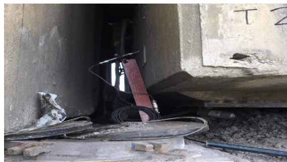
Figure 12. Damage of the Real-Time Transducer due to Excessive Movement
